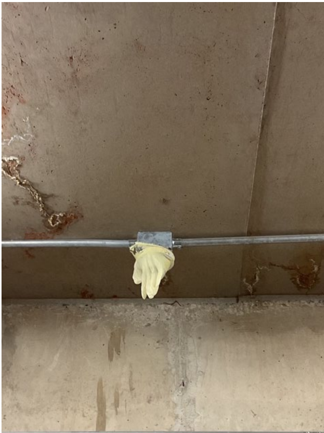
FIGURE 1 - IMPAIRED BOILER ROOM SMOKE DETECTOR
