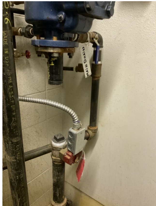
FIGURE 2 - MISSING FIRE SPRINKLER PIPING
