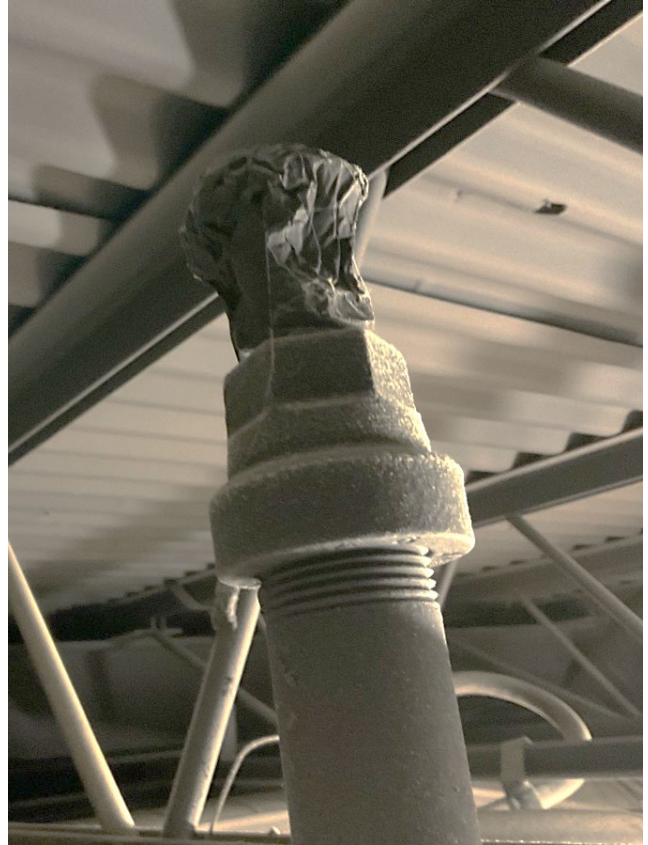
FIGURE 3 - COVERED FIRE SPRINKLER
