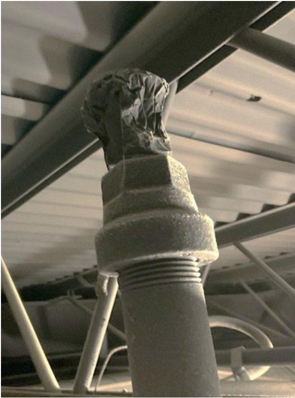
FIGURE 3 - COVERED FIRE SPRINKLER
