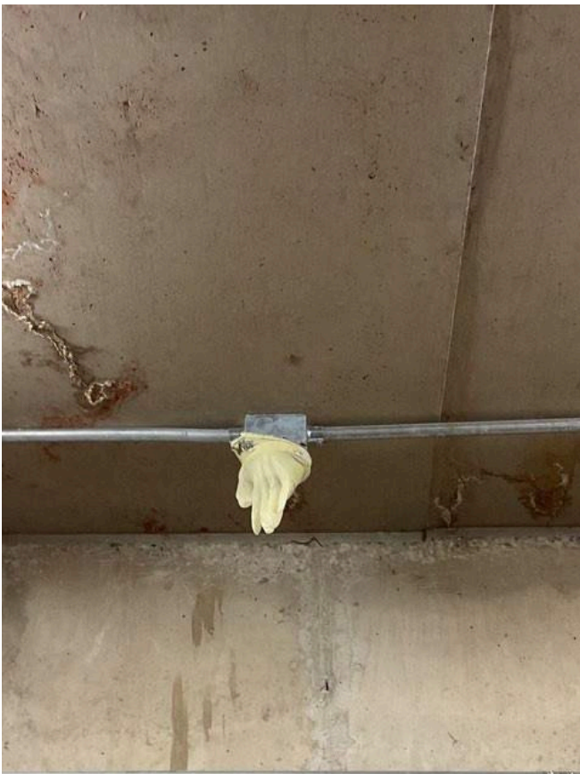
FIGURE 1 - IMPAIRED BOILER ROOM SMOKE DETECTOR
