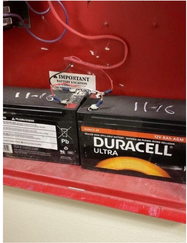
FIGURE 4 - CORRODED FIRE ALARM PANEL BACKUP BATTERY TERMINALS
